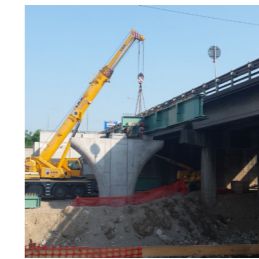
Brescia Ovest Brescia, Italy 2013
